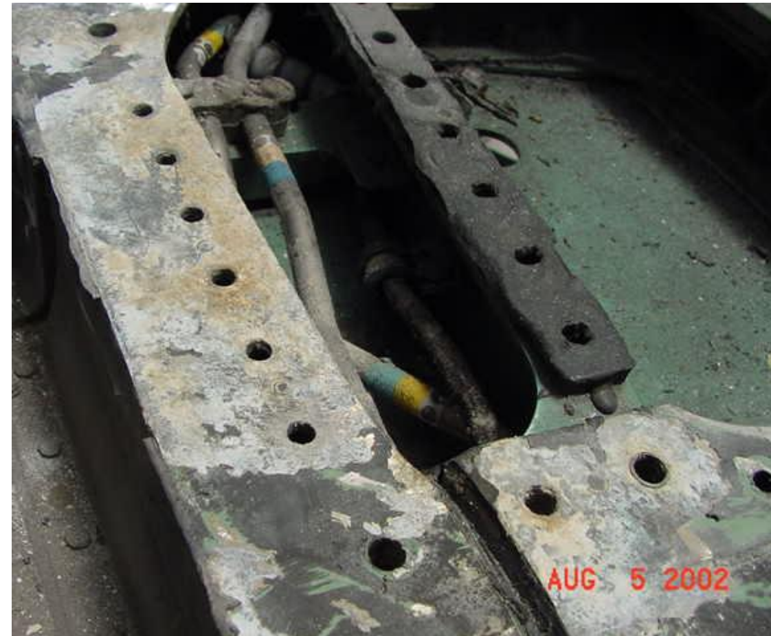
Repair: Remove corrosion and bush hole with PH stainless; now corrodes even faster around bushing, just as we predict computationally
